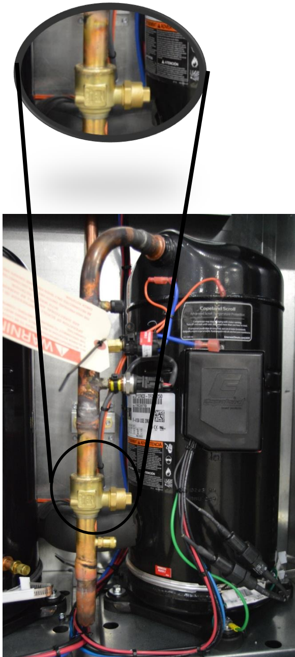
Figure 131 - Compressor Isolation Valve
