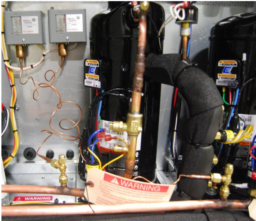
Figure 138 - Adjustable Fan Cycling Installed in a Split System Condensing Unit
