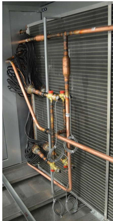
Figure 37 - EXVs in AHU
