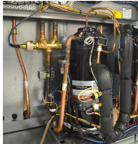
Figure 66 - Modulating Hot Gas Reheat 3-way Valve Installed in Condensing Unit
