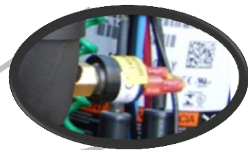
Figure 152 - Low Pressure Switch
