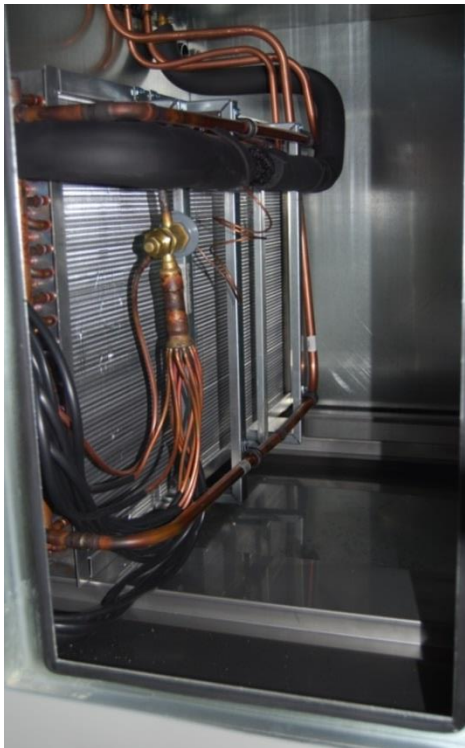
Figure 30 - TXV in Air Handling Unit
