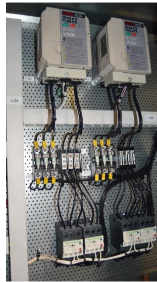
Figure 139 - VFD Controlled Condenser Fan Head Pressure Control
