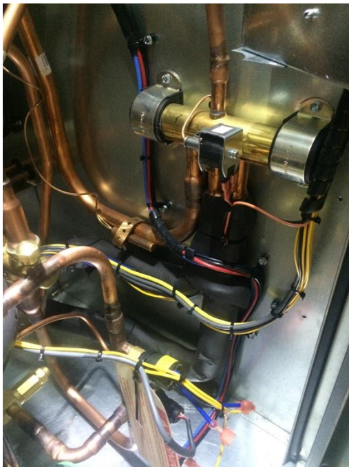
Figure 75 - Reversing Valve Installed in Condensing Unit
