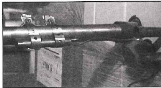
Figure 32 - TXV Bulb Installed on Suction Line
