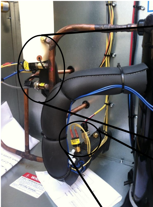
Figure 135 - Schrader Valves Installed on Discharge and Suction Lines
