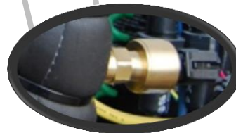
Figure 153 - Suction Pressure Transducer
